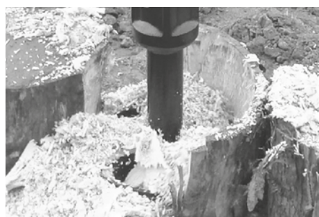
After the planer has cut deeply enough, just change the position and redo until the stump is completely removed.
