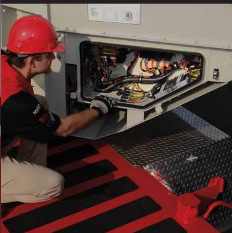
Illuminated upper electrical panel
